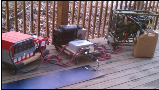
2.0 kW Hybrid Power System
