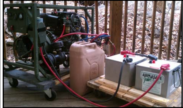
4.5 kW Hybrid Power System
